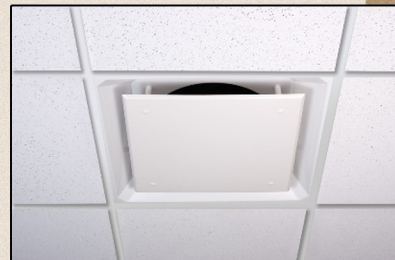
Air Diffuser / Air Return
